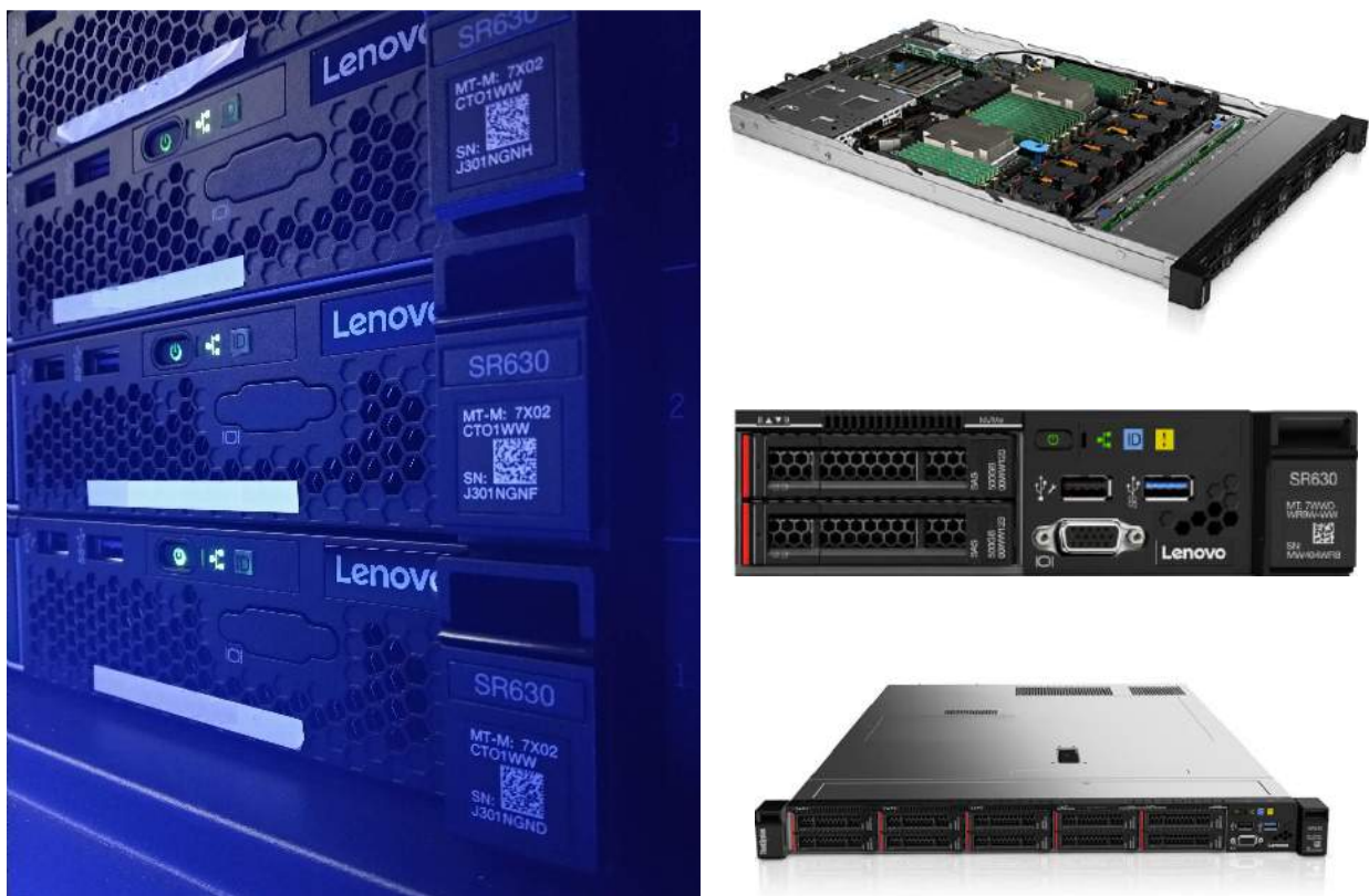
Figure 19 – SCAYLE Lenovo SR630 server
