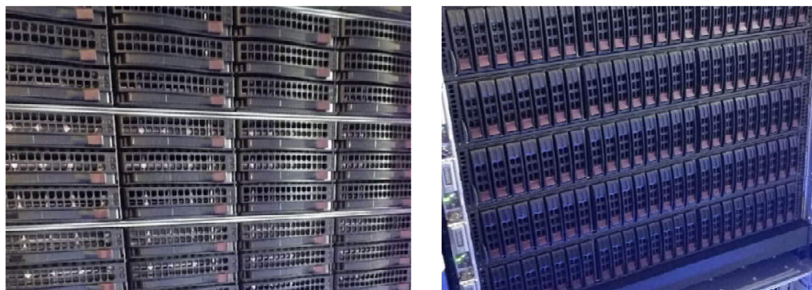
Figure 15 – Haswell SCAYLE infrastructure
